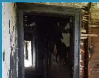
Fire Damage Restoration
